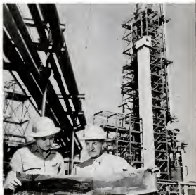
NEW TYPE "CAT CRACKER" goes up in a New York refinery. This modern development in oil refining squeezes more high octane gasoline and fuel oil out of each barrel of crude oil. To win more business with better oil products, oil companies are constantly improving manufacturing methods.
